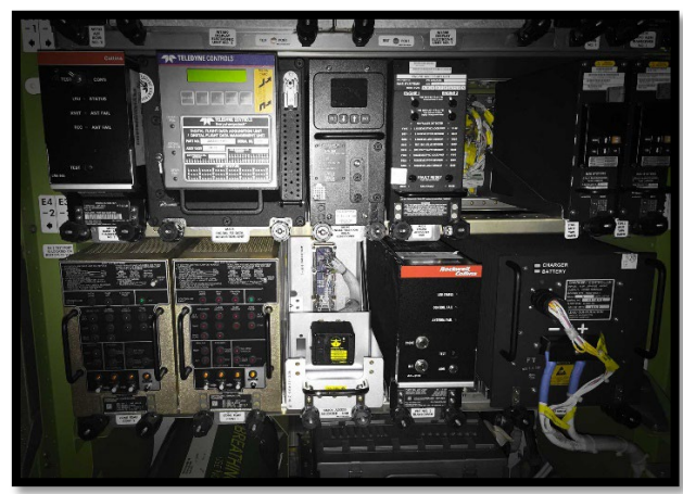
Figure 2 - E-Bay Install for QAR / DAR Data
