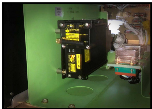
Figure 3 - E-Bay Install for Augmented QAR / DAR Data
